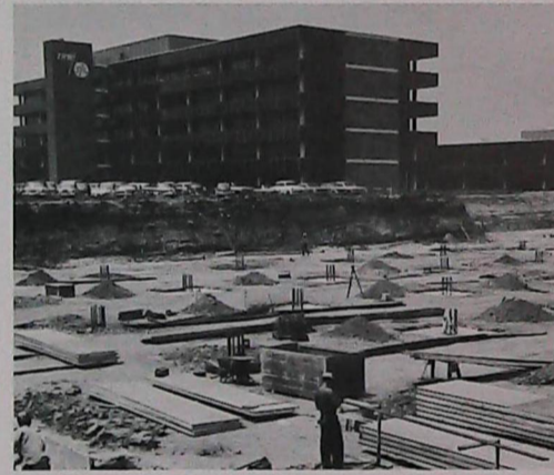
WHEN THE BASIC complex of Space Park was started, construction on new buildings soon followed. Pictured here is the beginnings of Building S. TRW employees have adjusted to the fact that construction is an on-going activity.
